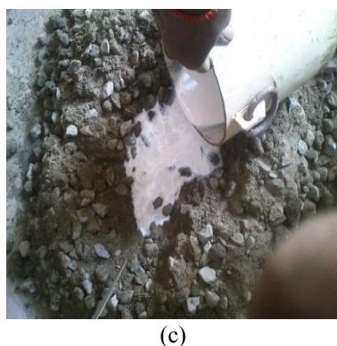
Fig 2.2 (a) (b) - SBR Polymer (c) - Mixing of the polymer in the concrete
